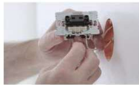
03 Connect the DALI PCU to the pushbutton.
